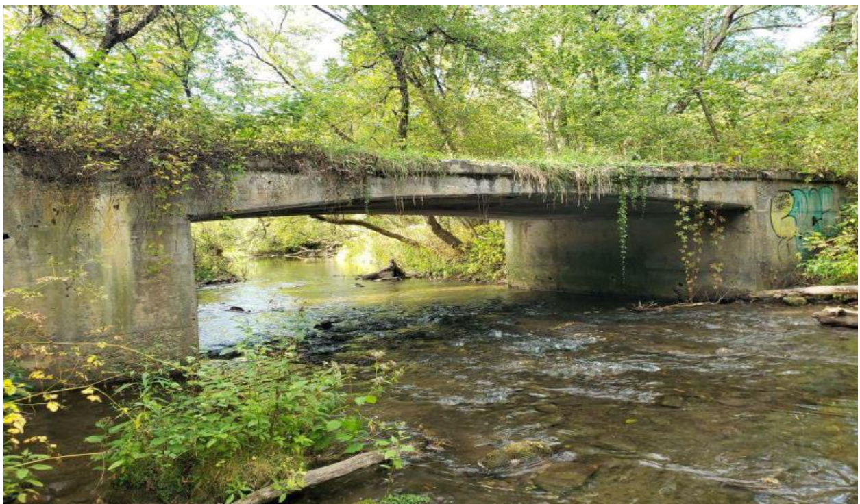
Figure 3.2: Example of Poor Condition Bridge – Norham Mill Bridge
